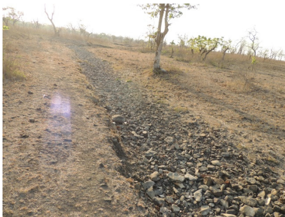
Figure. 3- Shallow stream due to soil erosion
